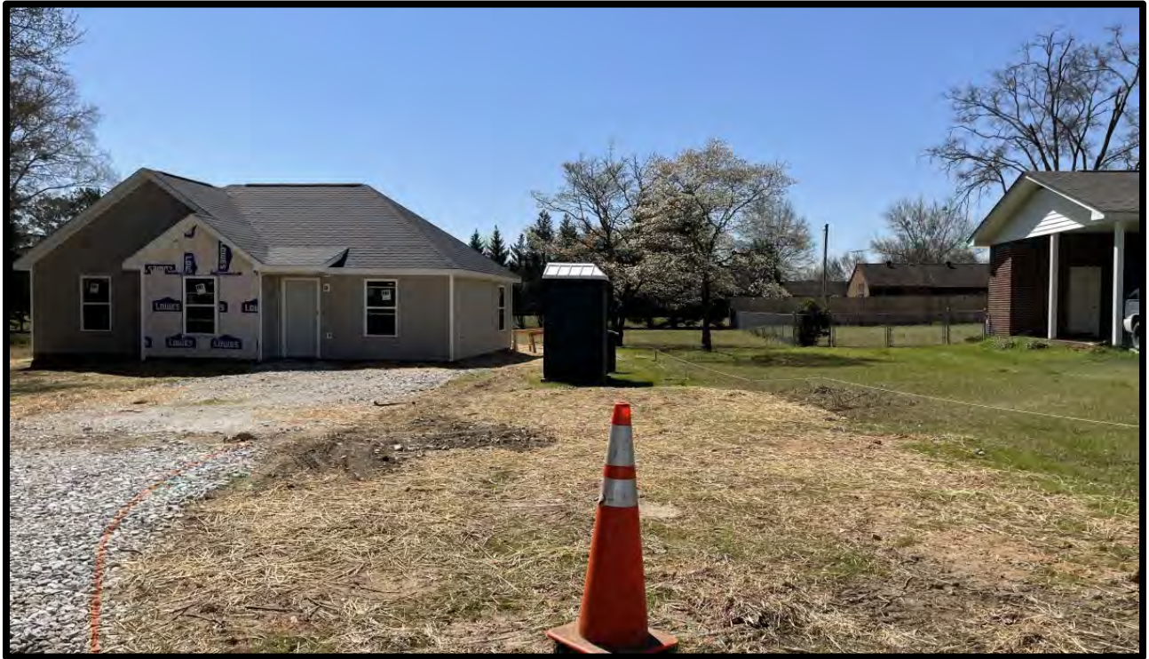
Photo 13—adjacent single family home under construction; the site is in the distance
